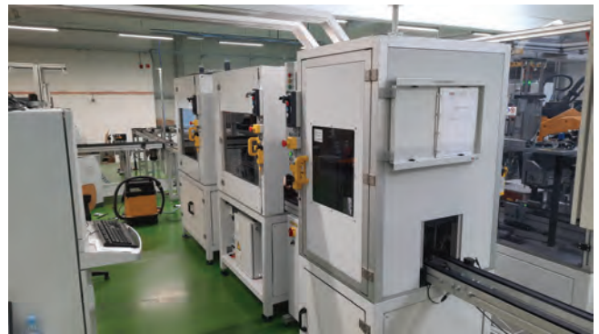
Figure 4: New diagnostic system for automatic final quality assessment of electric motors at Domel d.o.o.
