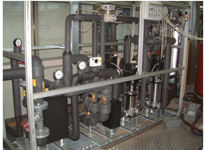
Figure 5. Semi-industrial setup for systematic functional testing of elements needed in the heating and climatisation of buildings. The control system for the setup shown here was developed by the Department of Systems and Control.
