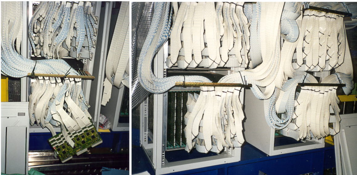
Figure 4.34: Two phases in the arrangement of signal cables on the front end driver system side. In the left side photograph the initial phase of cabling is presented. Also one front end driver daughter board with partially connected signal cables is seen, while on the right side photo, the final cable arrangement is seen.
