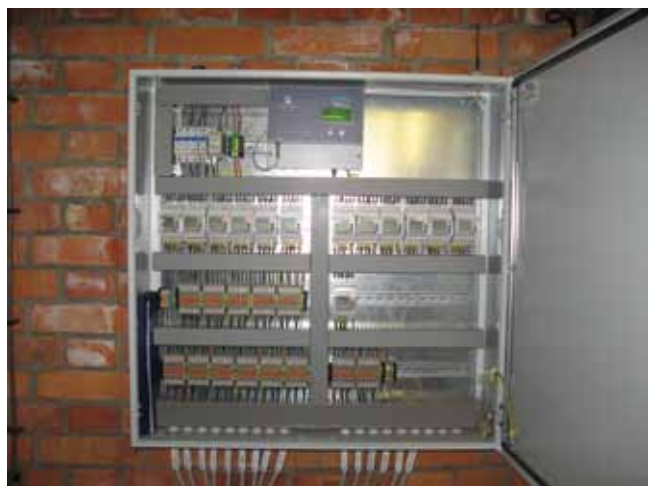
Figure 2: New installed measurement and communication equipment for monitoring electricity use in RCP JSI premises
